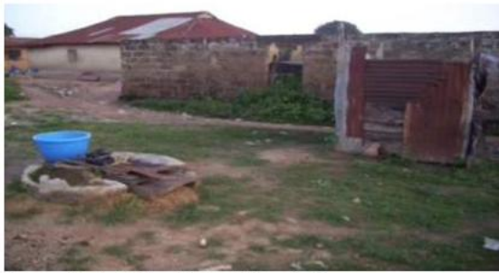
Figure 3: A Dilapidated Hand-Dug Well in Iwo Town
